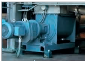
WANGEN KL-R pumps in operation
